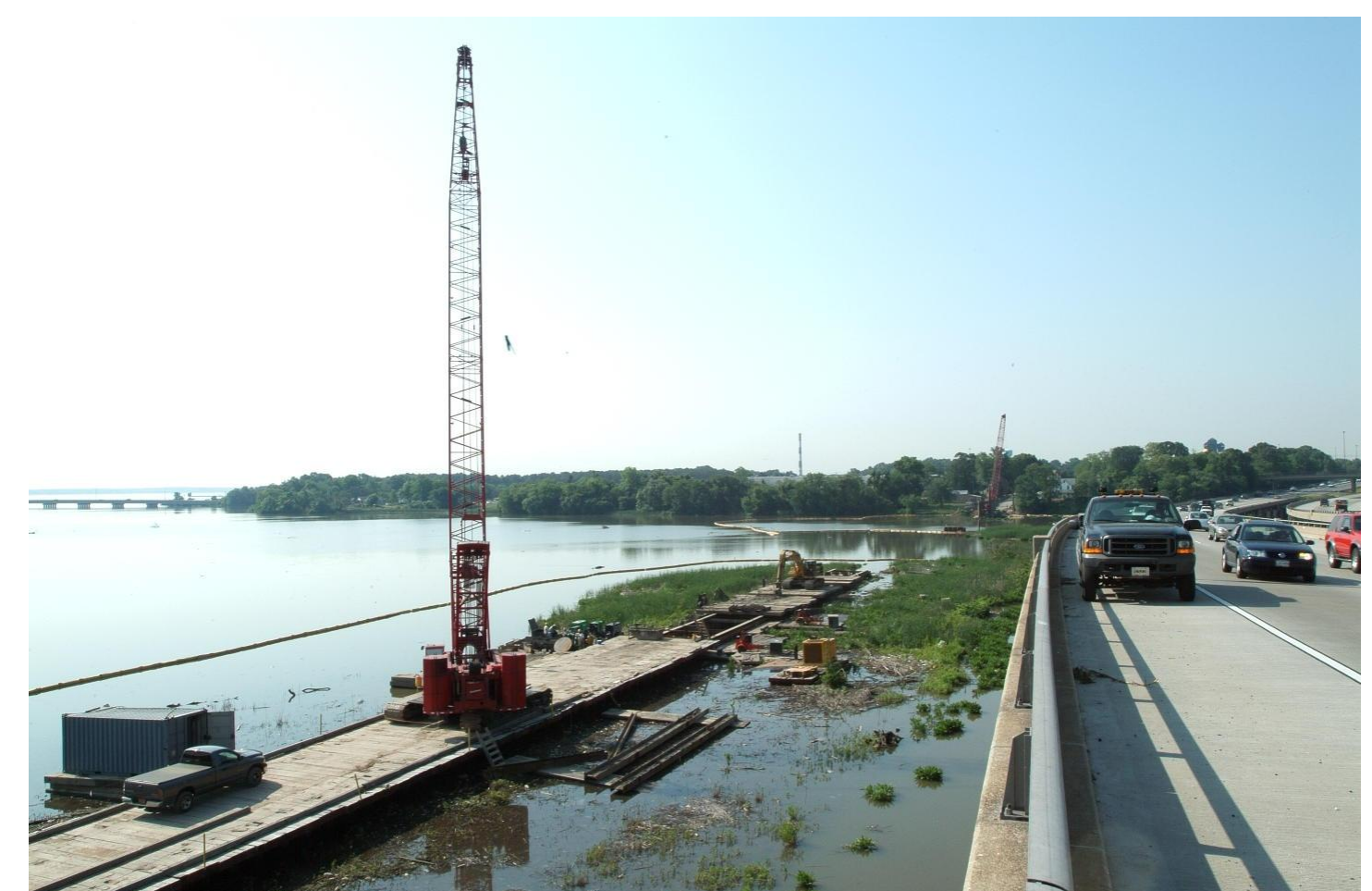
Pipe installation in the foreground with SSP installation beginning from the south shore
